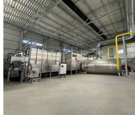
Waste water treatment plant, Constanta, Romania
